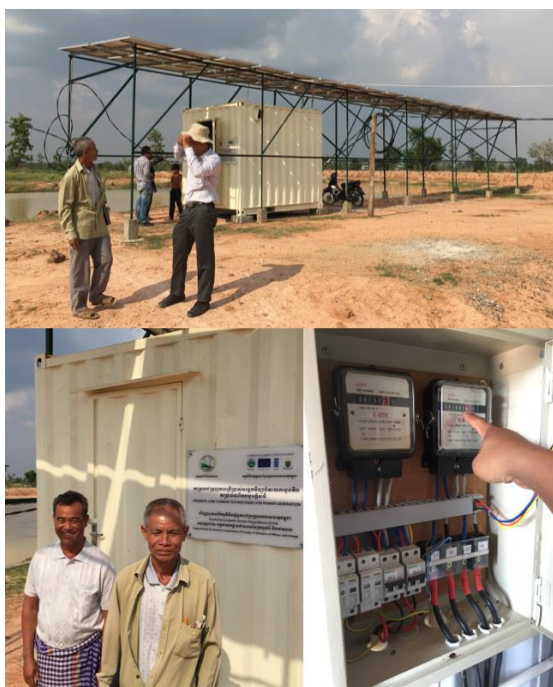
A MICRO-GRID SOLAR-BASED ELECTRIFICATION SCHEME MANAGED BY A COMMUNITY-BASED COMMITTEE IN PURSAT PROVINCE – MME PROJECT
