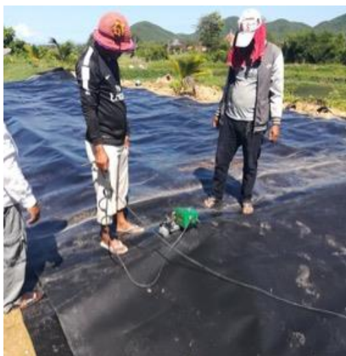
INSTALLATION OF PLASTIC LAGOON AS PART OF A MEDIUM-SCALE BIODIGESTER SYSTEM AT A PIG FARM – NBP PROJECT
